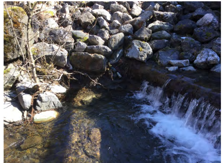
Log across stream is causing scour to riprap
