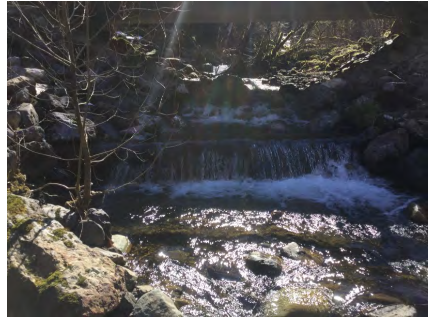
Log across stream is eroding and causing scour to riprap
